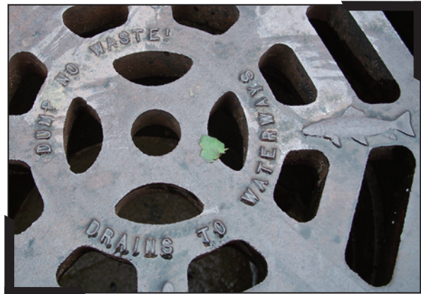
This storm drain is marked with fish symbols and text that indicates, "Dump No Waste! Drains to Waterways."
