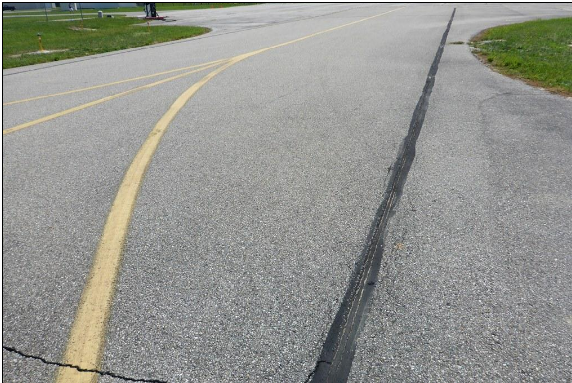
Figure 2-5. Typical AC Pavement in Fair Condition (Feature 310)
