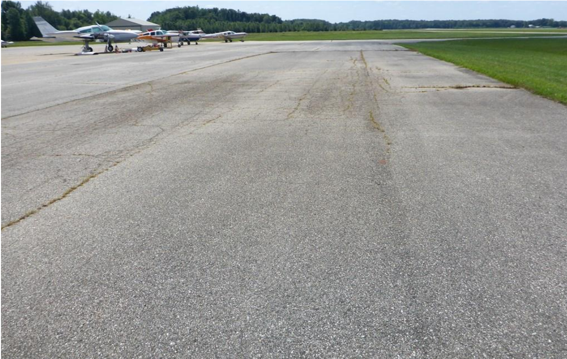
Figure 2-6. Typical AC Pavement in Poor Condition (Feature 3010)
