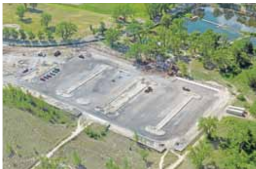
April 2012 saw the start of $1.5 million in improvements to two parking lots at Marquette Park. These included new water and sewer connections as well as lighting and sustainable features such as rain gardens to manage stormwater runoff.
