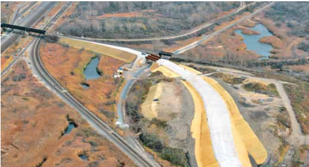
The Roland property as seen from the air in November 2012. Following soil compaction, two new rail bridges were built and the bed for the new rail lines laid (in white).
