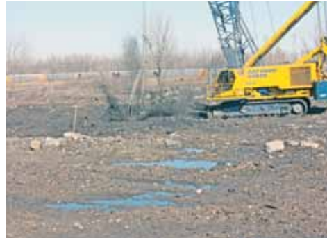
Work began early in 2012 on the former Roland property, which had been used as a dump for tires and construction debris. The land was cleared and the soil compacted by slamming it repeatedly with this 30-ton weight.
