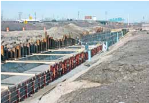
Workers in January 2012 constructing a box culvert in a drainage ditch between the airport and Cline Avenue. When the $5 million project was completed later in the year, it was covered over and the new rail bed built above it. (See photo at left.)
